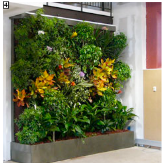
Living Wall installation, Baltimore, MD. This 110 sq ft (10 sq m) wall filters all the air for its 7,500 sf office building. Notice the ornamental character of some plants chosen
